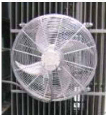
Figure 9.16 Transformer Cooling Fan
