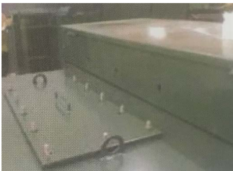
Photo 1. View of handhole installed on transformer tank cover
